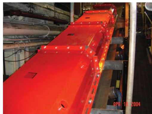
Figure 2 - transfer point containment
